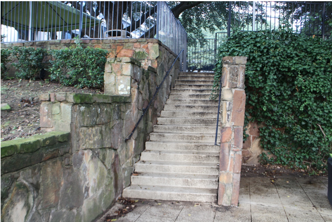
Photo 13: Typical steps and retaining walls at amenity area looking northwest. Photographed by Jay Firsching, December 2019.
